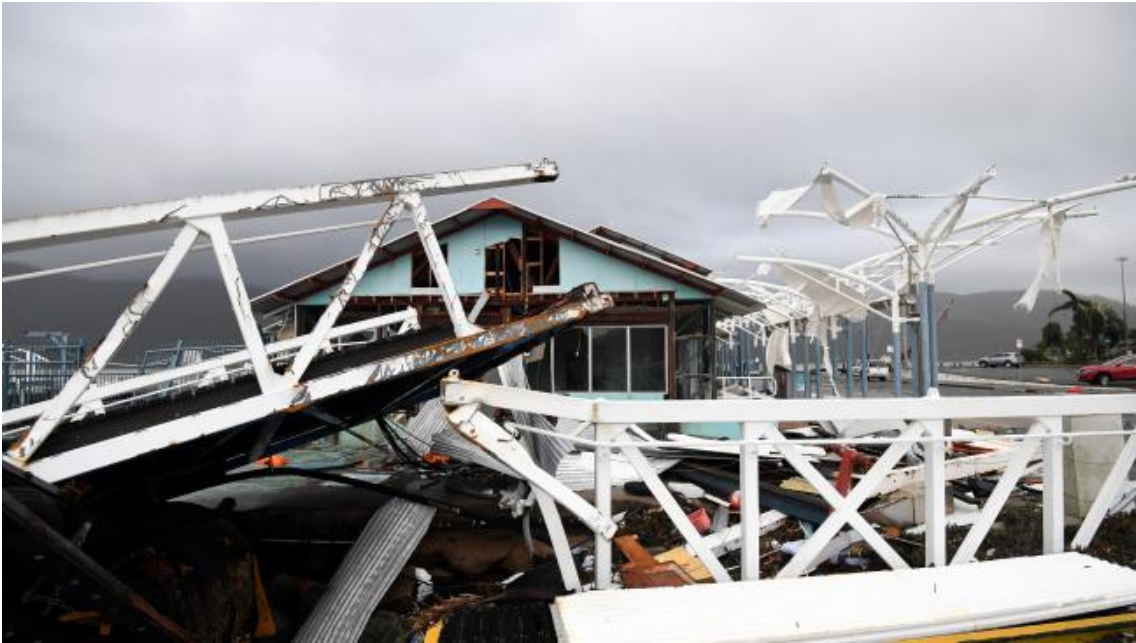
Severe damage to a boat terminal at Shute Harbour, Airlie Beach. Picture: AAP.Source:AAP
